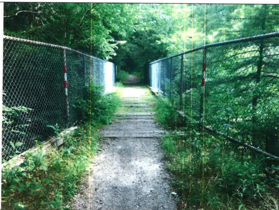
Photo 22. This old railroad bridge over Jabish Brook appears to be in good enough condition to accommodate pedestrian traffic and maintenance equipment.
