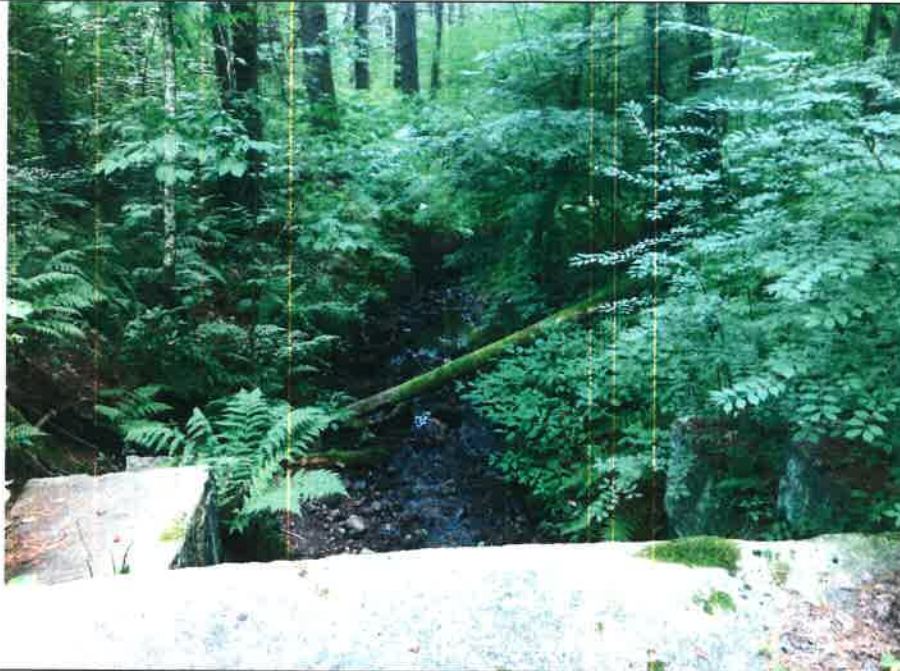
Photo 25. Not far from Route 181 is this stone culvert, which appears to be in good condition.
