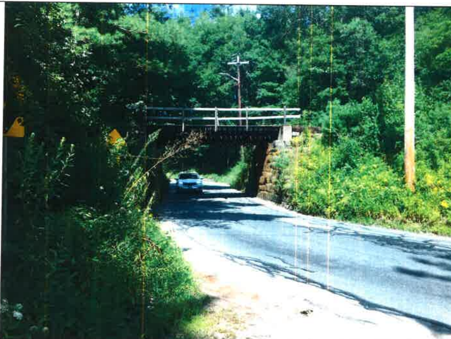
Photo 30. View of the North Washington Street railroad bridge and its stone abutments from the south. This bridge has a 30-foot span, but because there are no existing abutments for an adjacent, future rail trail bridge, its span would need to be 50 to 80 feet in length. A fiberglass pedestrian bridge might be the best option here.
